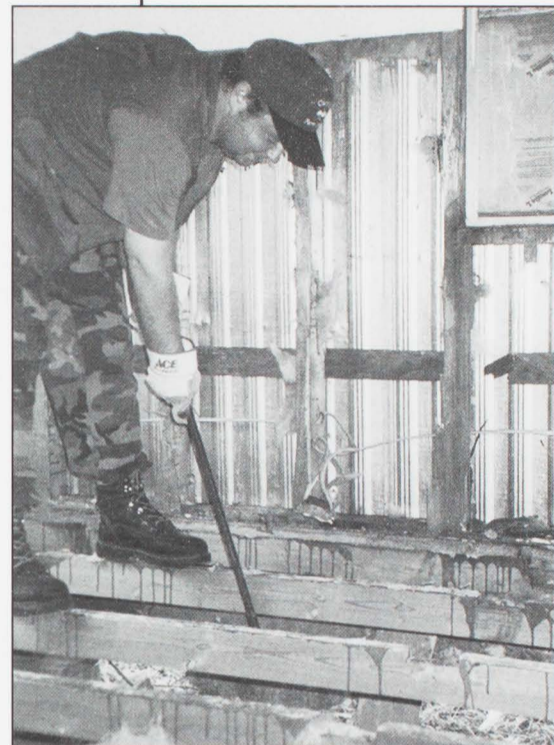
Britt Fisher, M.Div. '02, uses a crowbar to pry up sub-flooring in a home near New Bern. Flood waters reached halfway up the walls.
