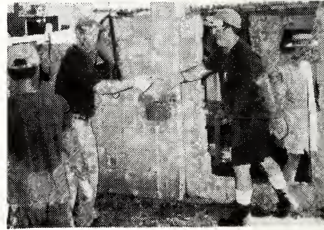
Wayne King and Phil Former passing the cement for the floor of the parsonage.
