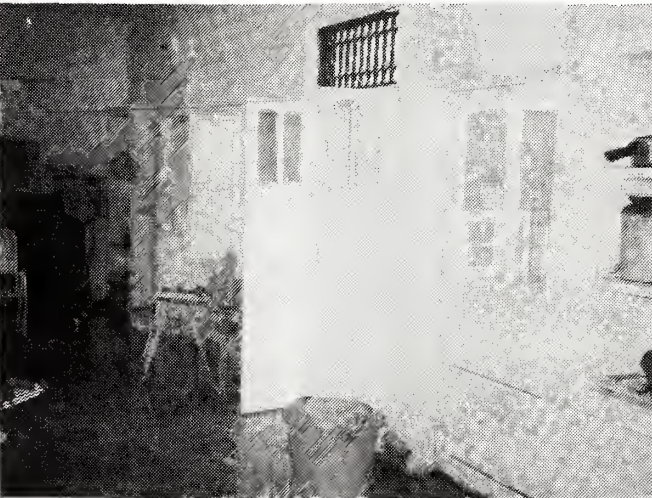
Inside view of the room that was restored after it was destroyed by fire.
