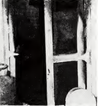
Room in Dr. Lall's home that was destroyed by fire.
