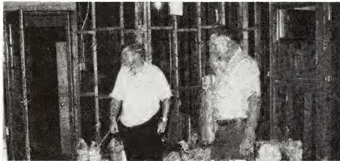
Mike Irvin is seen inside his home after the interior has been removed, with the exception of the wall studs. Drying-out time takes six weeks. Also pictured is the Rev. James Owens.
