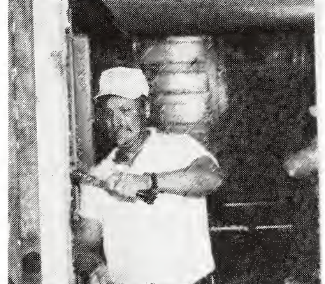
Phil Armstrong constructs the new doorway connecting the new education building to the existing sanctuary at Mt. Tabor FWB Church, Creswell, NC
