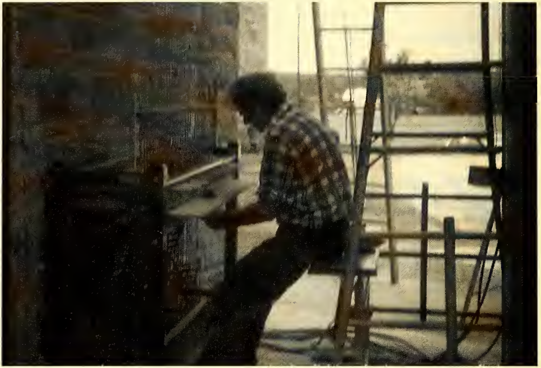
Installation of the carillon, 1972–1973. The 1895 cornerstone was lost behind the carillon, only to be rediscovered in 2000 when the carillon was renovated.
