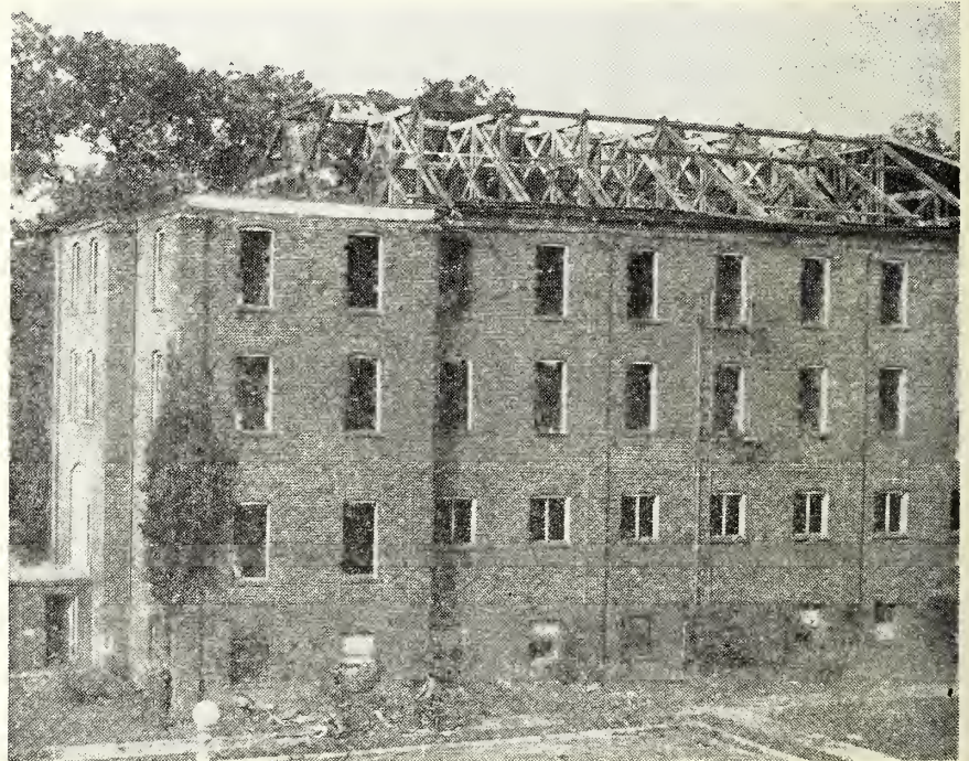
The old gymnasium at Elon is finally coming down. This view is from the third floor of Alamance. Beneath the vine at the corner of the gym is Pres. J. Earl Danieley who is talking with two young boys on bicycles. The boys have just discovered that the roof of the old landmark is gone.
