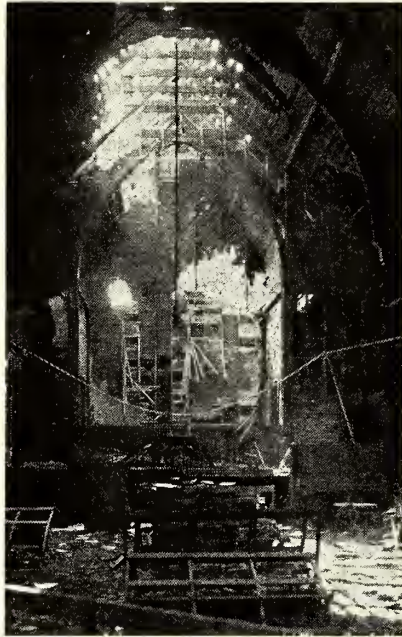
Fire Damaged Church of Wide Fellowship Southern Pines, N. C.
