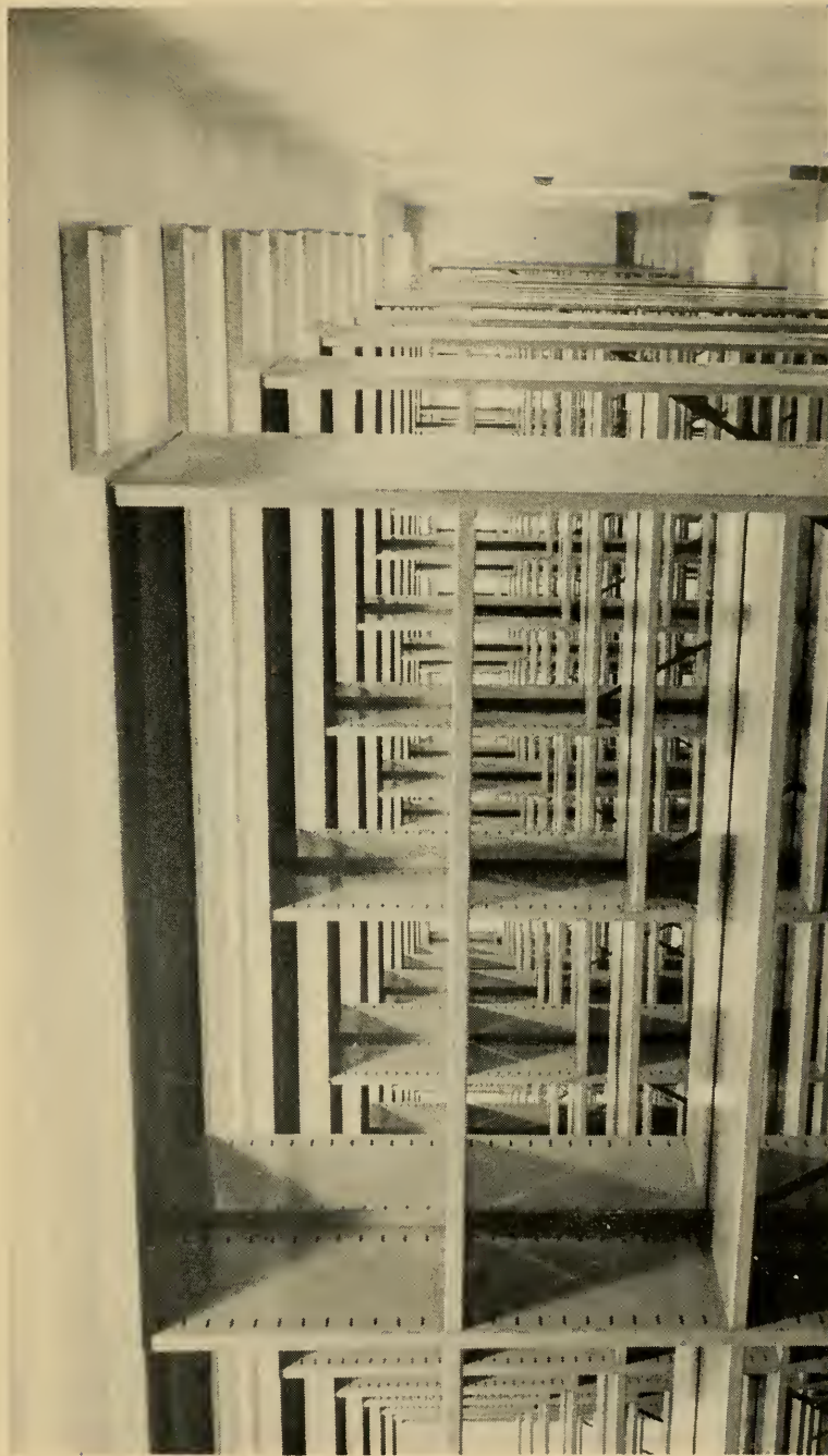
The new library-stacks. This is not the boiler room of the Queen Mary but the space for the expansion of the library facilities. It will hold 50,000 volumes, which the faculty hopes will be read.
