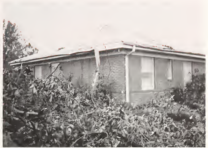
The roof of Cannon Cottage at the Pre-Adolescent Center was damaged when a large tree fell on it. Other damage occurred to roofs on Howard Cottage at the Adolescent Center, the gymnasium, a two-story storage building, and several campus houses and apartments.
