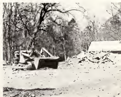
SPRUNT INFIRMARY is no more. Demolition workers remove last vestiges of a once outstanding building which had served well. Think of all the mumps, measles, bandages, splints, whooping cough, etc. etc. etc. new history. With the gifts of two brothers, James Sprunt and William H. Sprunt of Wilmington, N. C. this structure was built in 1916.
