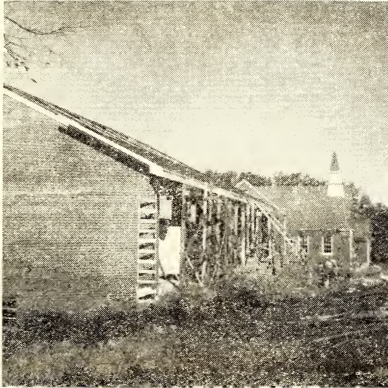
ROOF IS ON MEMORIAL BUILDING, this picture shows work to date on the memorial building. It is hoped that it can be completed at an early date.
