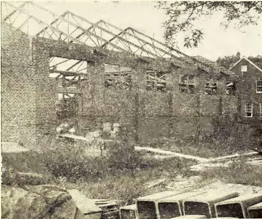
ROOF NEEDED BEFORE COLD WEATHER to cover Johnny Luke, Jr. Memorial building.
