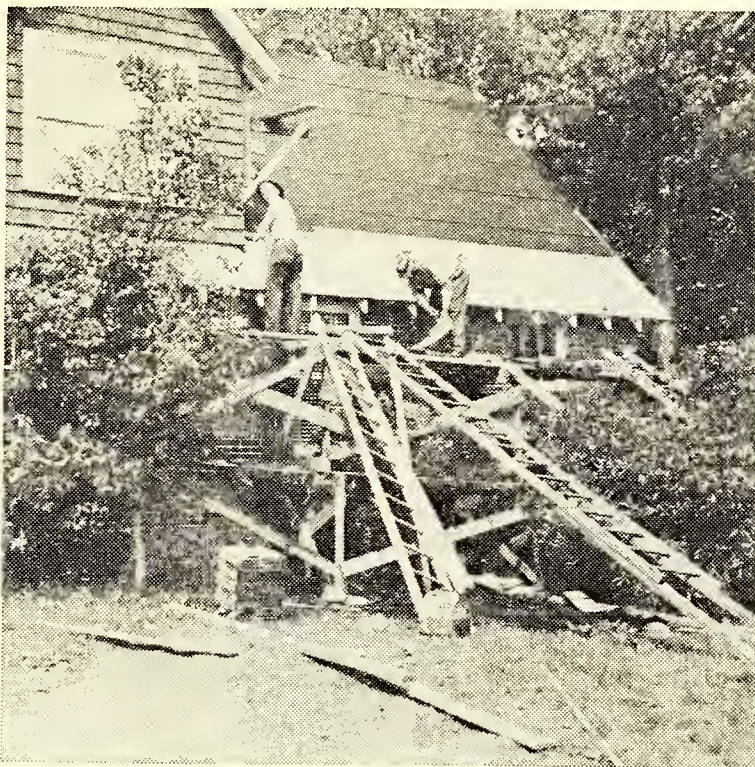
THESE MEN are hard at work putting a new roof on the Glendale Springs manse.
