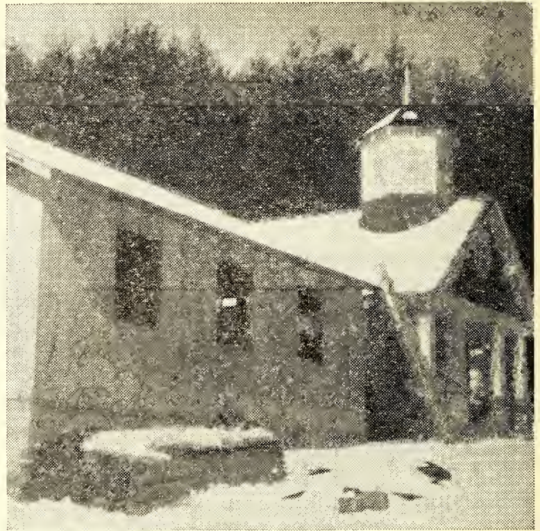
WORK PROGRESSES on the Sunday School addition now being built at Laurel Fork Presbyterian Church.
