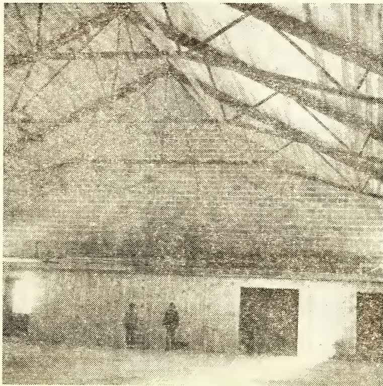
INTERIOR OF MEMORIAL BUILDING is needing to be completed and work is hoped to go forward soon.
