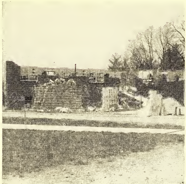
CONSTRUCTION IS GOING FORWARD on new building for boys at Glade Valley. This will replace the building which was destroyed by fire. (News Photo)
