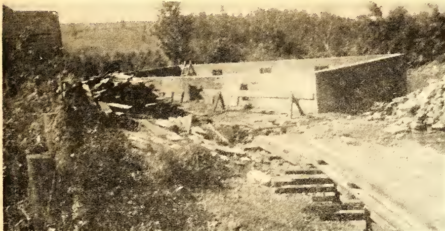
Workmen have been busy on the new church building for Ebenezer Presbyterian church. Here is a view of the foundation for the new church building.
