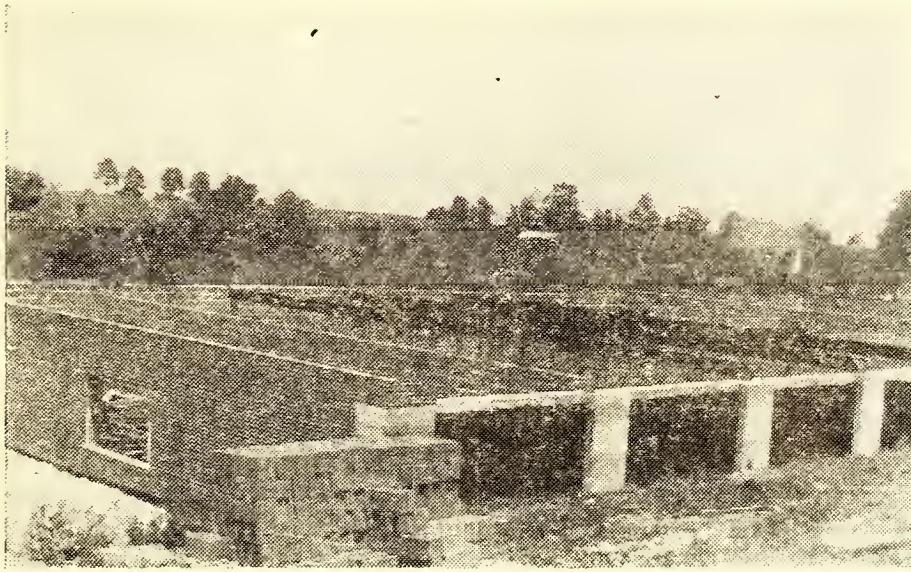
HALF WAY MARK IS REACHED on the Johnny Luke, Jr. Memorial building, where more funds are needed.
