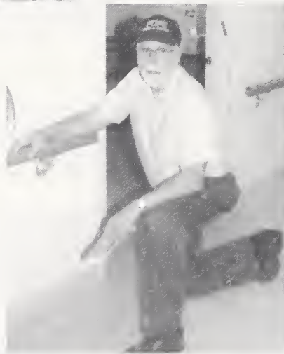
Jesse Clauson, of the maintenance staff, can be seen putting a new face on the A-wing corridors. A cheerful teal blue now greets visitors to A-wing and brightens residents days.
