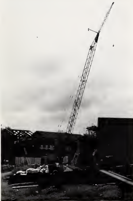
Using this crane, workmen position each steel beam. At left is two-story addition to B-wing which will house dining rooms and elevators. At right is back side of Commons.
