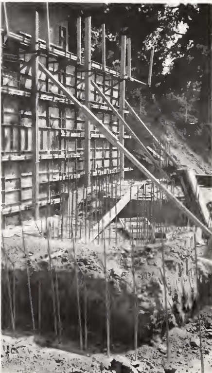
Below: At the east end of A-wing a wall goes up where the connecting link will meet A-wing and the Commons area.
