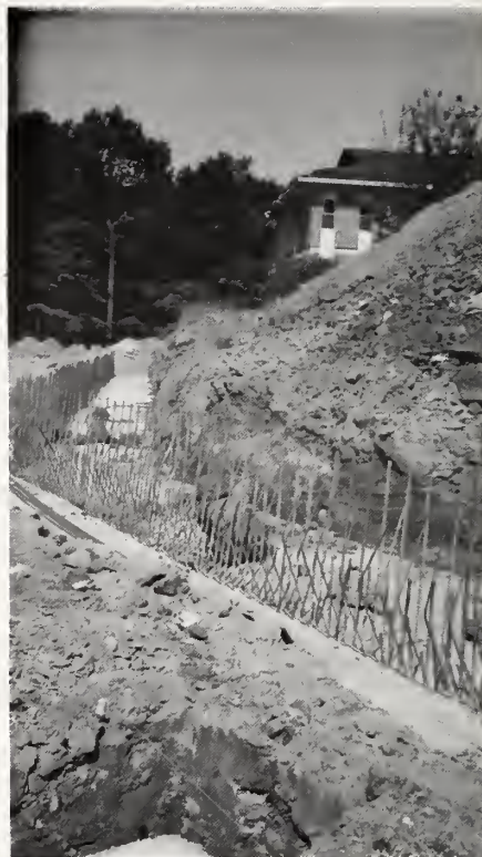
Above: Steel spikes mark the route of the future gallery — passageway between A- and B-wings. A new crafts shop will be housed there also.
