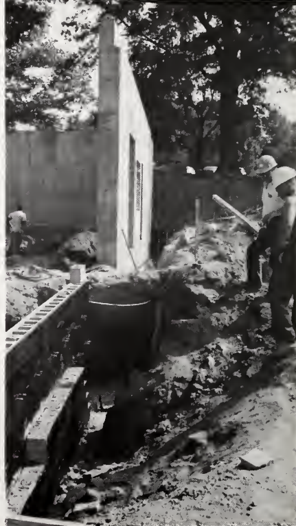
Below: Workmen surveying the basement foundation of the Commons, where the new kitchen will be located.
