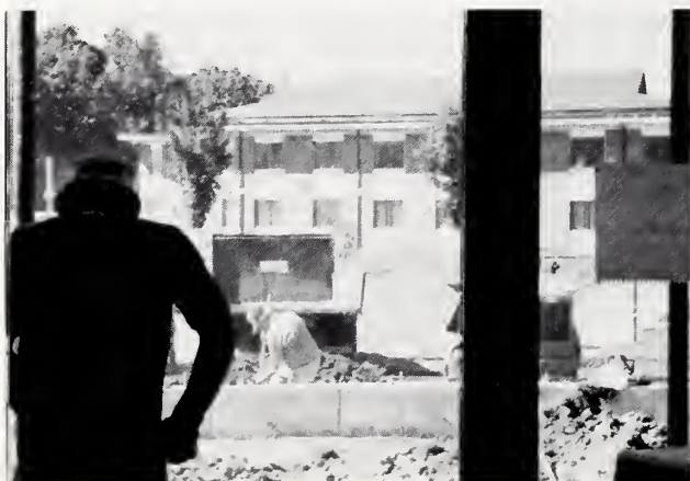
Construction on A Wing continues. Since this picture was taken, the walls have been built!
