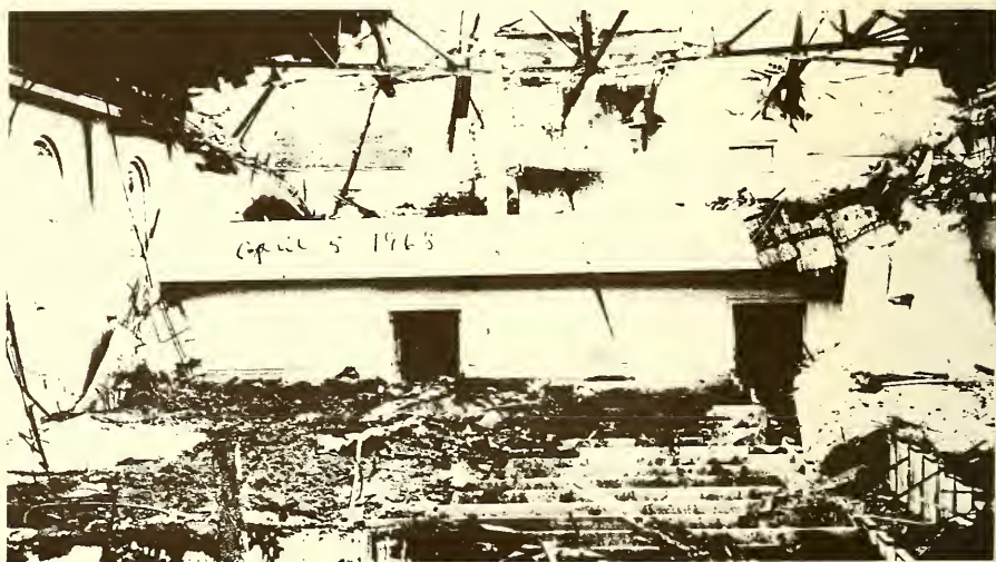
DAMAGE caused by an early morning fire at Balfour Baptist Church today is indicated by this photograph taken after fire-fighting operations had ceased. The scene looks toward the rear of the sanctuary
