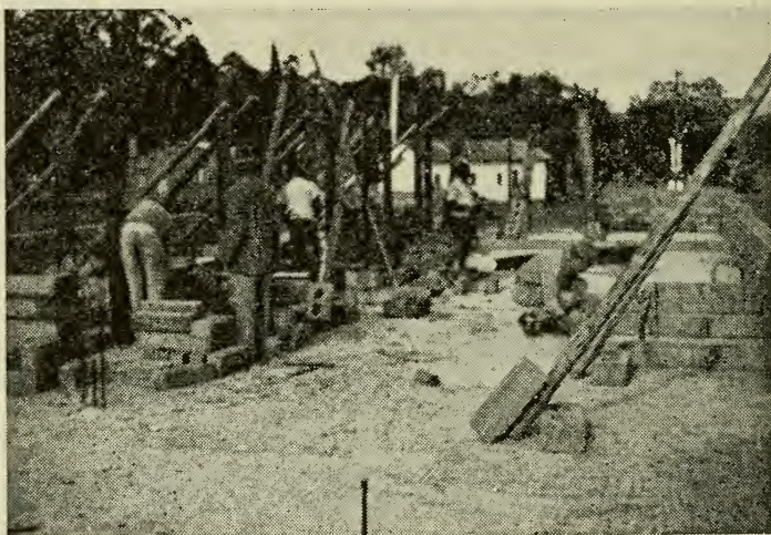
Mr. Everett Matzigkeit measures during the construction of the new press building. Mr. Wallace Sithole of Nyamuzuwe was the contractor.
