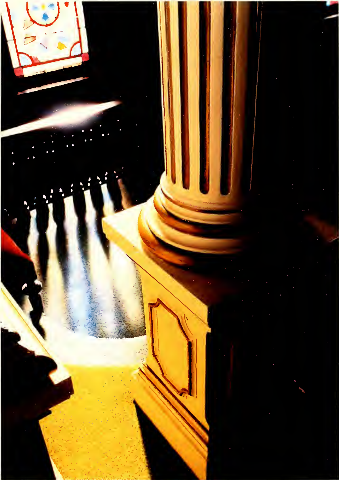
Close-up detail of the column base. The light through the stained glass creates interesting patterns on the floor.
