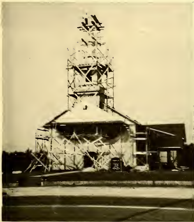
Pastor Walton is on top of steeple. It is about 70 feet high - the cross makes it 80 feet. The cross was put into the top the next morning (June 24, 1957), J. O. Walton, Roger Sharpe & Paul Kesler placed the cross into its place. Roger Sharpe went 4 feet higher than Paul and I, dropping it in. (written by Rev. J. O. Walton, v. G.)
