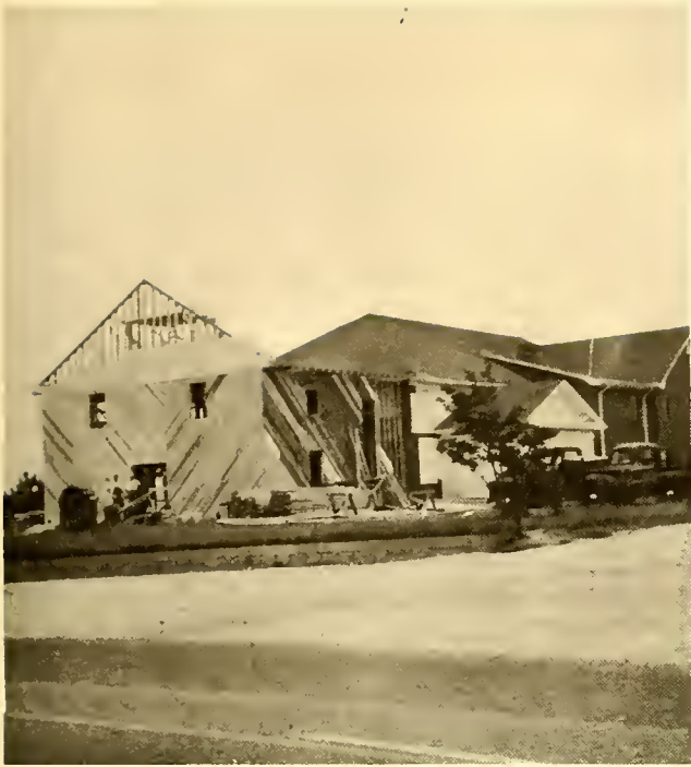
Beginning the second month's work (June 1, 1957). First rafter is set up; storm sheathing is put on front. Picture taken from Mr. & Mrs. K. W. Greene's yard.
