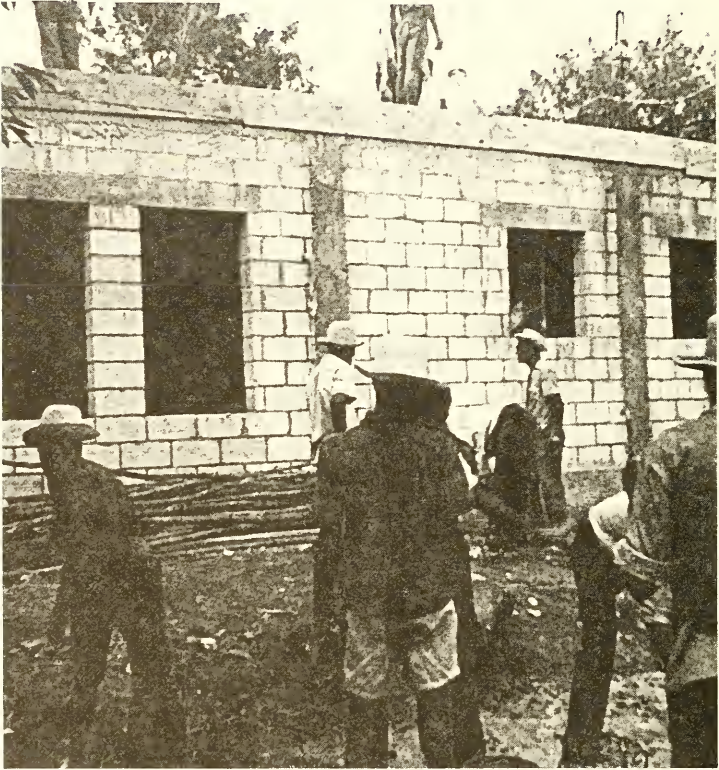
Figure 13.1 View of typical building team activity. Workers are constructing a religious training camp residence at Camp LaHatte in Haiti, West Indies
